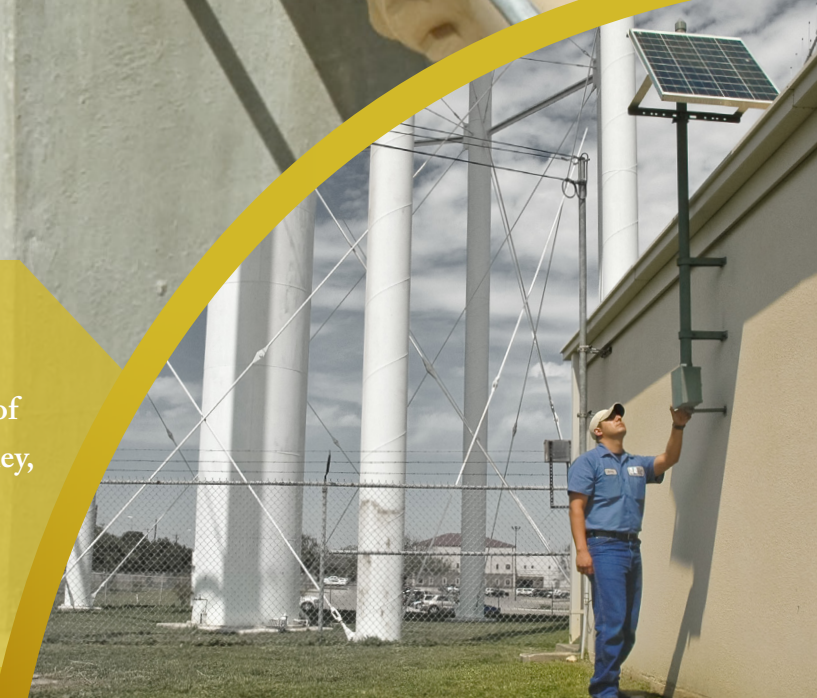
Newly installed solar power system cuts energy costs for SAWS.
